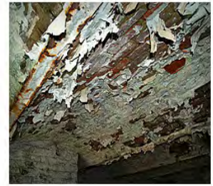
Peeling paint from builder24car
